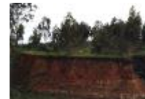
The government planted Eucalyptus trees along the edge to prevent further erosion. They found out that the root system actually caused further erosion.
